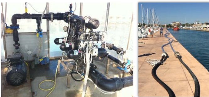
Portoverde filtration system
